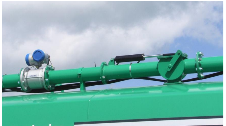
Figure 3 Flow Meter and Control Valve
