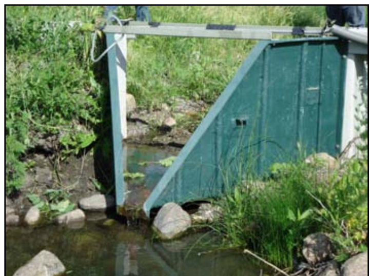
This flume at the Amanns’ second collection site is equipped to measure water flow and obtain samples for nutrient testing.
