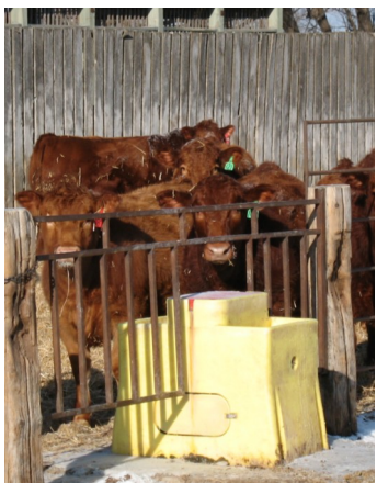
An insulated and heated watering system for cattle.
