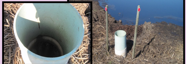
This solid separator is no longer functioning. The corrugated pipe is plugged and dirty water is backing into the feedlot. The solid separator should be dredged and cleared of plant growth.
