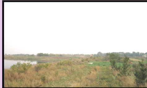
This manure storage structure needs vegetation management. The grass should be mowed, and trees and shrubs should be removed from the inside bank and from close proximity to the structure.
