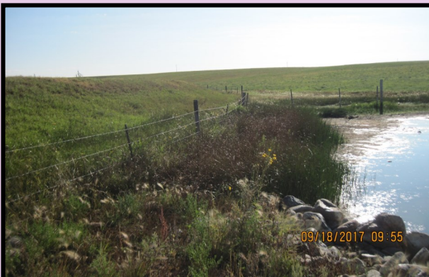
Rip rap has been placed at the base of this manure storage structure to reduce the potential for erosion.
