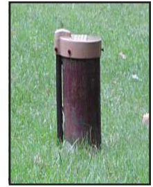
Common well head for a 4-inch diameter casing with submersible pump.
