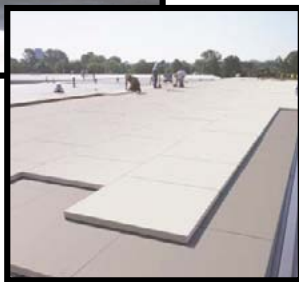
Figure 5. Continuous insulation on roof deck. (Courtesy of U.S. Department of Energy building codes university)
