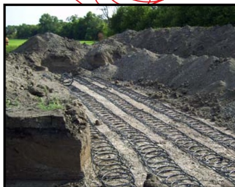
Figure 10. Loops for ground source heat pump. (Dennis Wiesenborn, NDSU)
