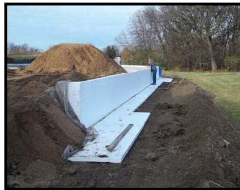
Figure 7. Frost protected shallow footing foundation for heated slab. (Courtesy of Larry Mayer, Solution Design Inc.)
