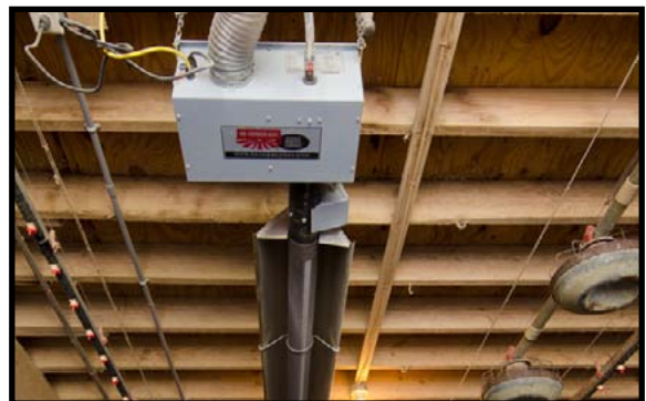
Figure 2. Radiant heater. (Courtesy of www.USDA.gov )
