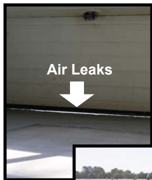
Figure 4. Air leaks resulting in wasted heat. (Carl Pedersen, NDSU)
