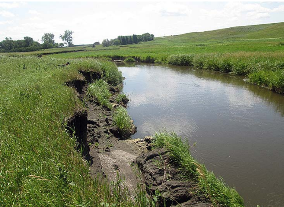
Bank sloughing along stream reach where riparian species have been replaced by smooth brome, resulting in widening of stream channel. (Miranda Meehan, NDSU)
