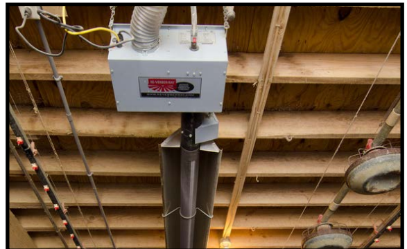
Figure 2. Radiant heater. (Courtesy of www.USDA.gov )
