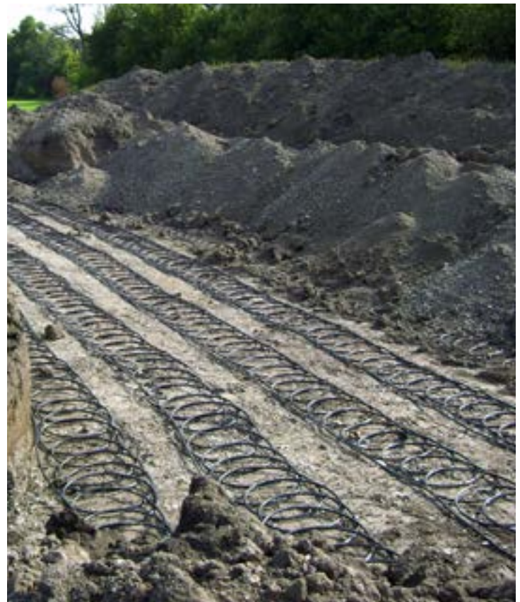
Figure 5. Horizontal ground loop (after)
