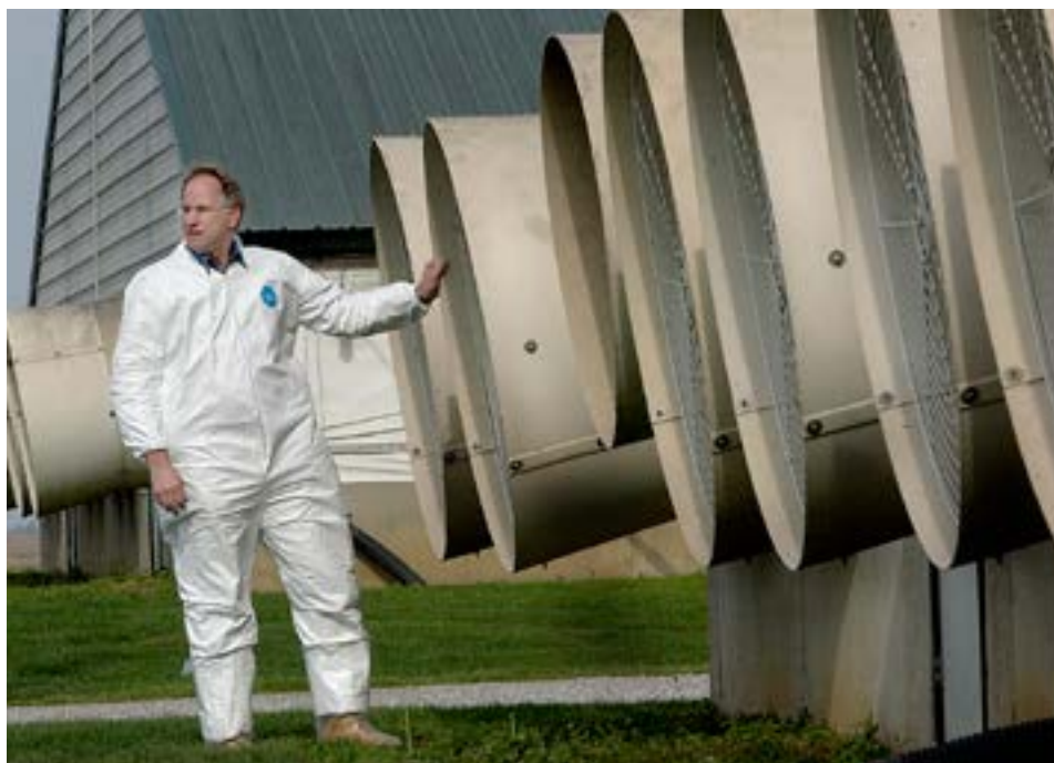
Figure 9. Livestock air ventilation system.
