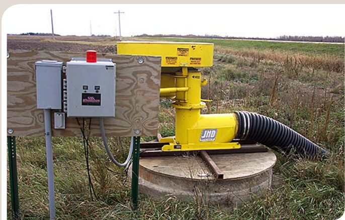
Figure 4. A concrete casing with metal cross beams supports the weight of the pump in this drainage lift station. This lift station also has a wooden cover with an access door. (NDSU photo)
