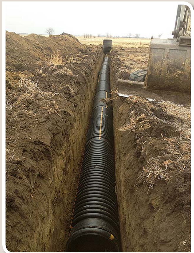
Figure 9. Two-foot-diameter corrugated plastic tile provides horizontal storage. (Photo courtesy of Ranger Pump Co., Vesta Minn.)
