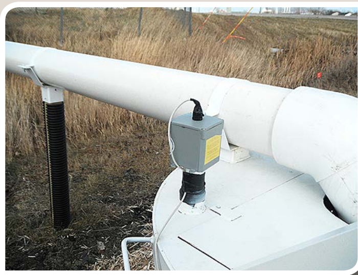
Figure 10. A pressure transducer box and pipe are part of this VFD-controlled pump. (NDSU photo)
