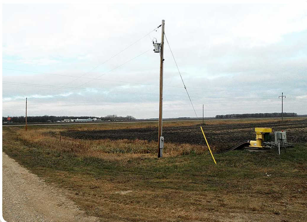
Figure 1. A tile drainage pump station is near power lines. (NDSU photo)
