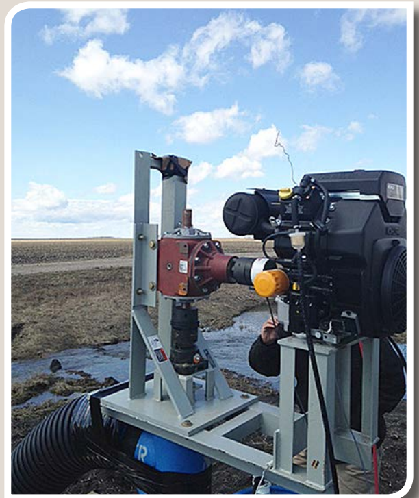
Figure 14. This engine powered drainage lift pump is controlled by water level sensors in the sump.
