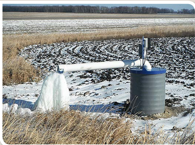
Figure 3. This drainage lift station uses a manufactured plastic sump casing with a metal cover containing a submersible pump. This photo was taken in mid-November when the temperature was below freezing. (NDSU photo)
