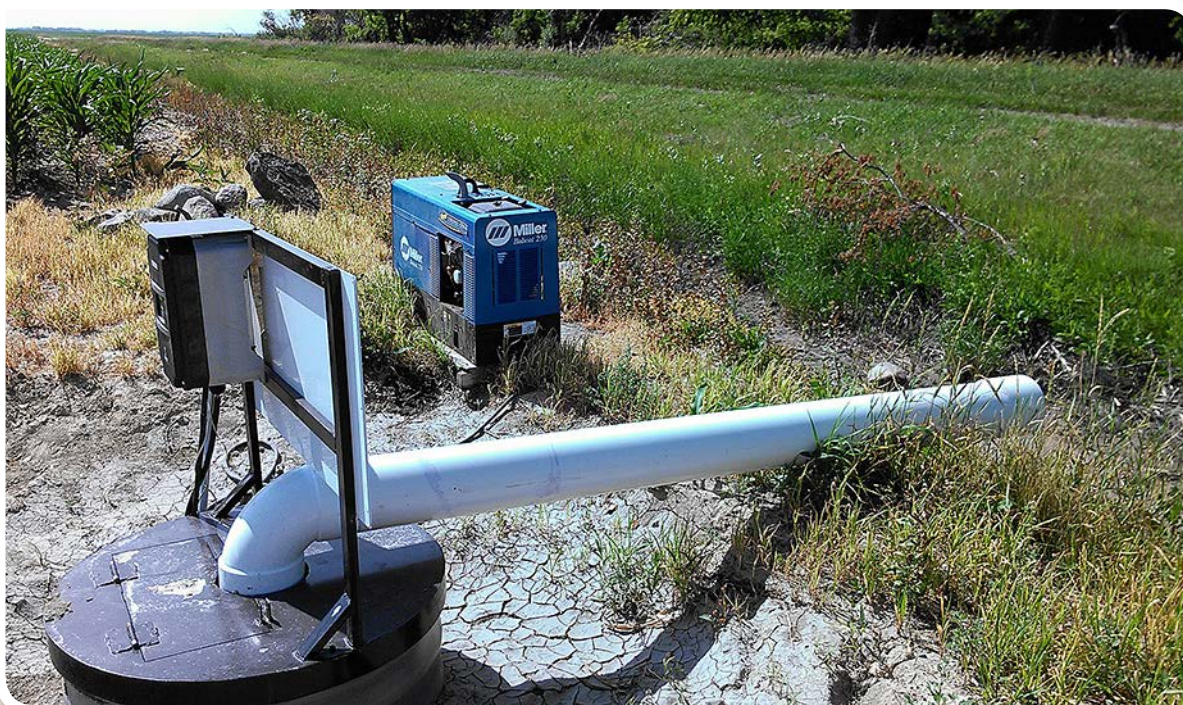
Figure 13. A generator is used to power the VFD-controlled submersible pump in this drainage lift station.
