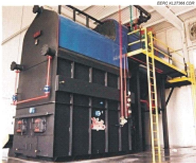
Figure 8. Hurst solid fuel-fired boiler (Hurst Boiler & Welding Co., Inc., 2006).
