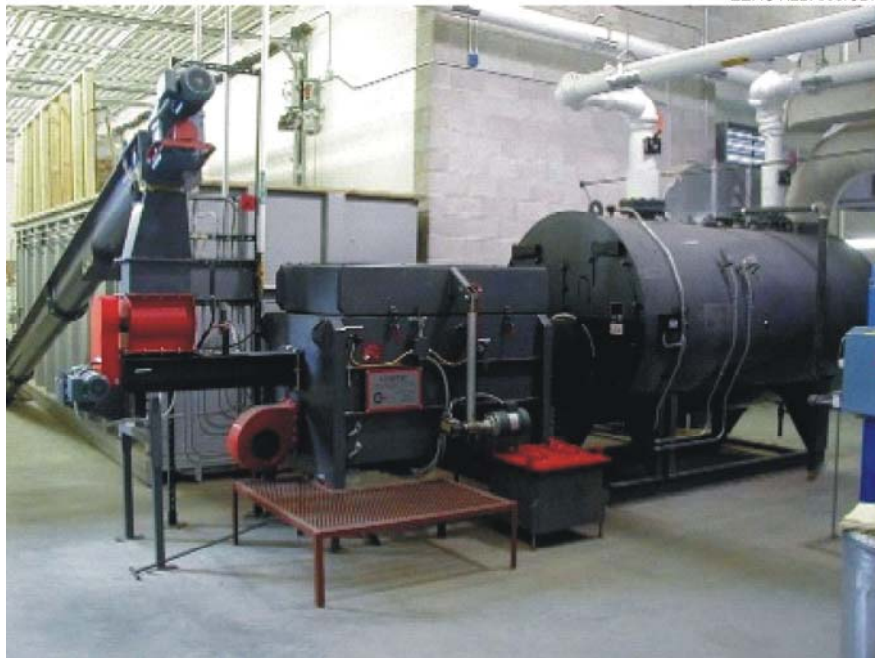
Figure 12. Chiptec gasifiers and boiler system (Chiptec Wood Energy Systems, 2006).
