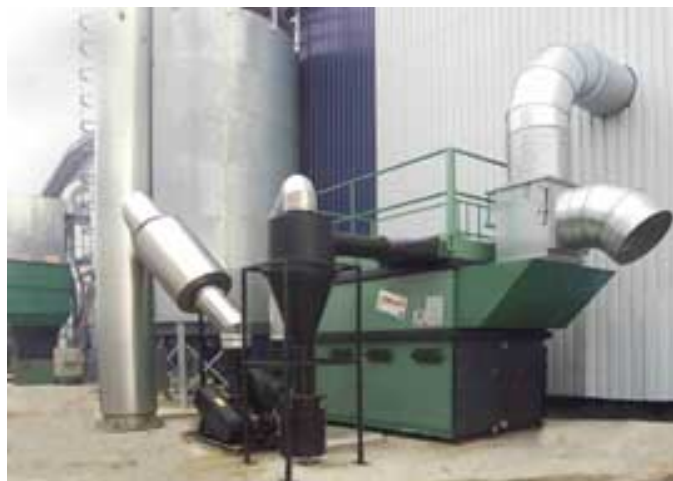
Talbott's 'C' Biomass System
