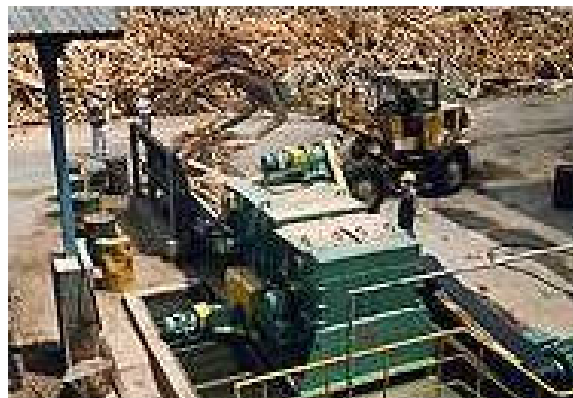
WSM Model 4048BHI Processing Slab Wood into Boiler Fuel in Malaysia
