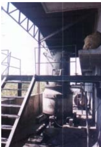
Gasifier Model: WBG-150, Mahabhadra Industrial Gases, in Operation Since 1994
