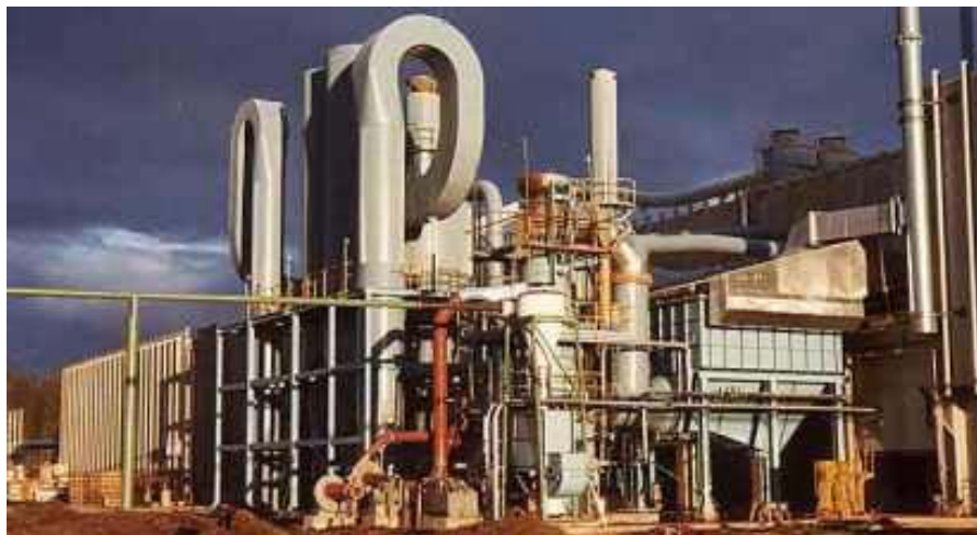
15 MMBtu/hr Unit in New Zealand
