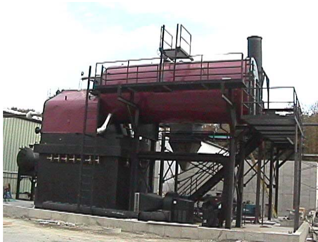
750 hp, 300 psig Wood-Fired Boiler System Installation
