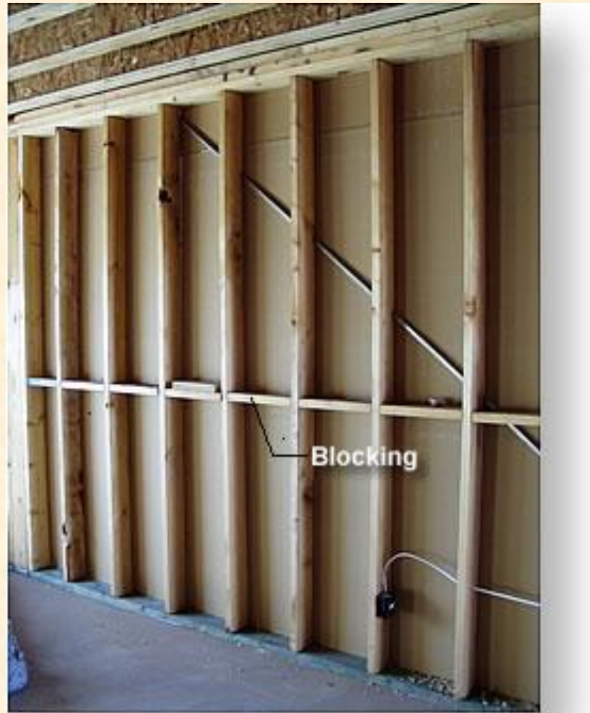
This is a 2x6 wall with a metal strap brace, treated base plate, and blocking.
