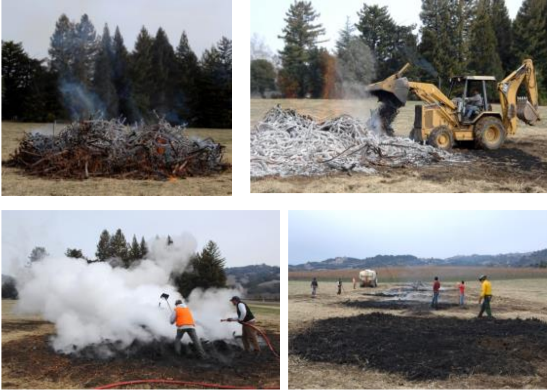
Figure 7. Once the pile collapses, it is time to tend and consolidate it. Quenching uses a combination of water and spreading to cool the char. If the char is not spread out, residual heat can evaporate all the water and re-ignite the char. Photos: Raymond Baltar/Sonoma Biochar Initiative.
