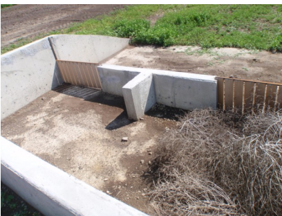
A maintained and cleaned out solids separator.
